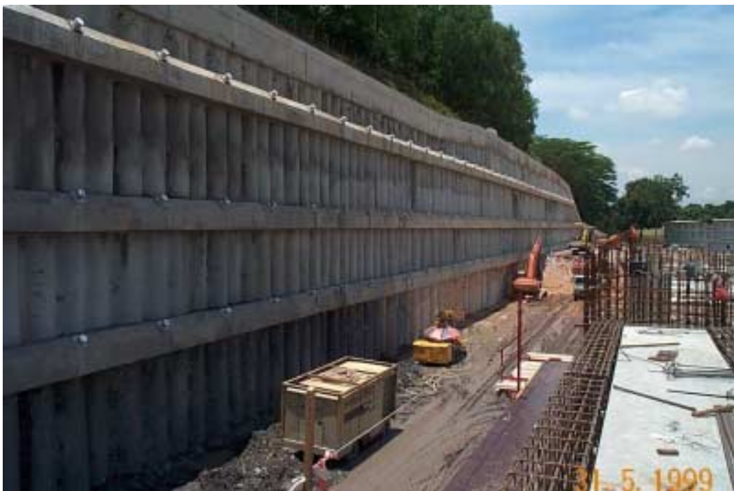
Photograph 4. 150-tonne working load anchors allowed the original number of 80-tonne anchors to be reduced by half.
