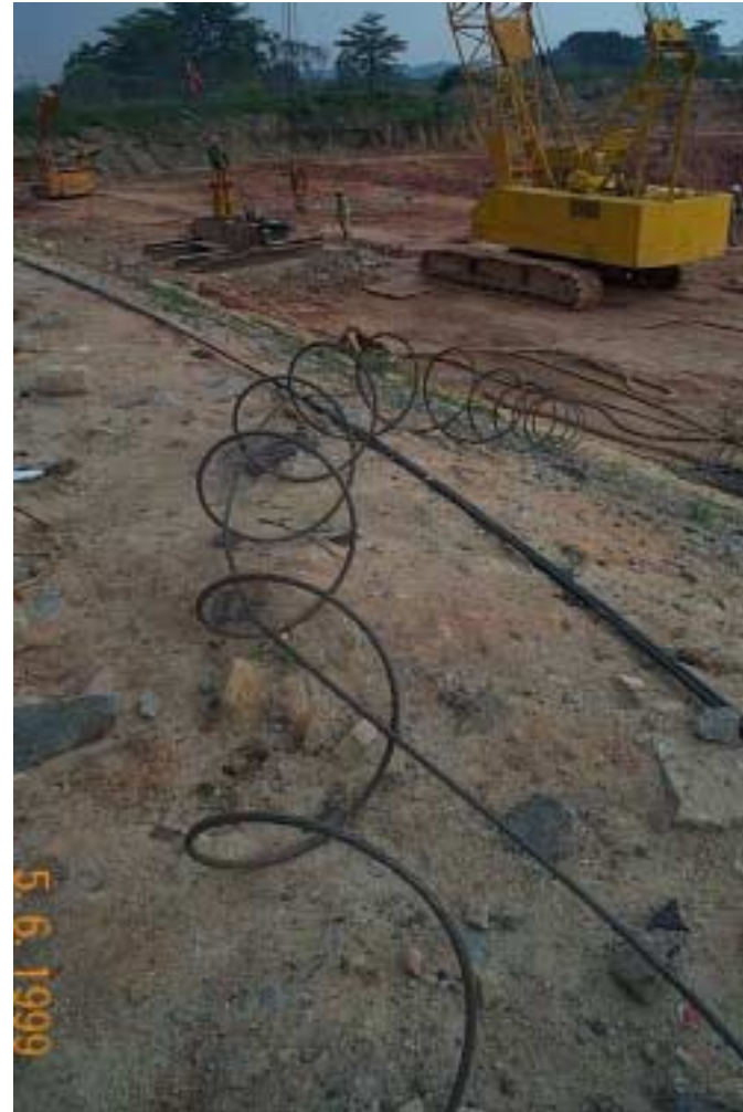
Photograph 2. Extracted strand of a removal anchor.
